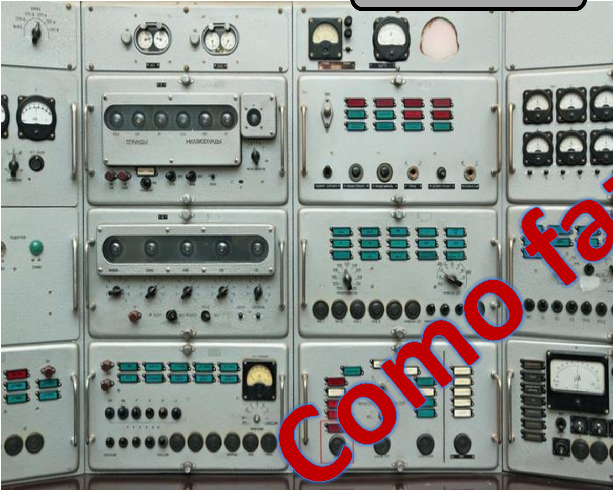
Painel de controle
